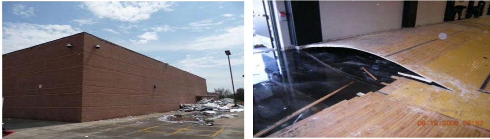
Figure 1 RICOWI, Inc. 2007. "Hurricane Ike Wind Investigation Report." Roofing Industry Committee on Weather Issues Inc., Powder Springs, Georgia. The flashing system became disengaged from the cleat, the fully adhered EPDM membrane did not peel back, but still allowed enough water to come through the header of the wall.
