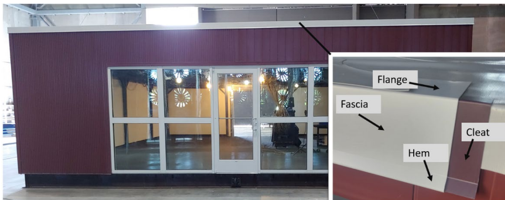
Figure 2 Flashing systems are composed of two layers: the interior cleat (maroon in the picture) and the exterior portion (white) which is broken up into three parts. The hem section connects to the cleat by tensions, the fascia section extends vertically down the wall of the building, and the flange section runs horizontally along the roof and is held down by fasteners.
